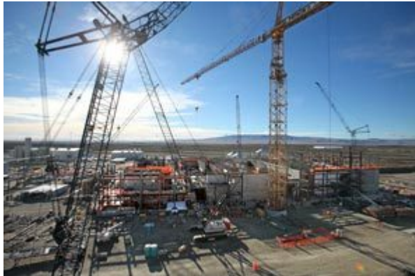
STEVE RINGMAN / THE SEATTLE TIMES Construction of Hanford's $12.2 billion plant to turn nuclear waste into glass takes shape in the desert outside the Tri-Cities.
